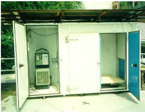
Plate 1. The dehumidifier dryer
